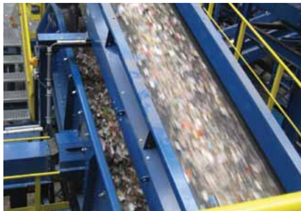
After being sorted by size, multiple conveyor belts take the lightweight packaging for further sorting.
