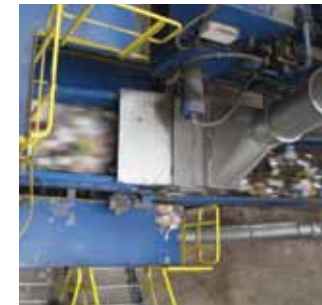
As a first sorting step, air suction is used to remove film plastics before they can bind the sorting equipment.
