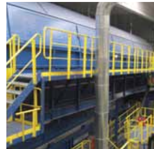
A view of the sieve drum (trommel).
